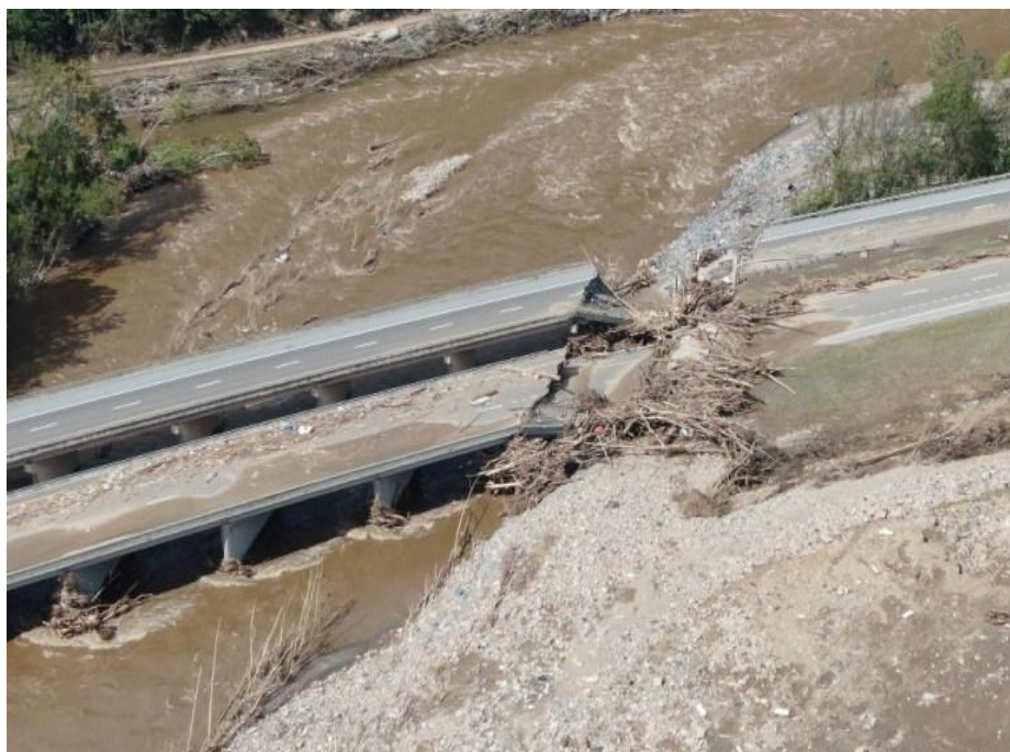
Interstate 26 bridge in Erwin, TN; between Johnson City, TN and Asheville, NC
