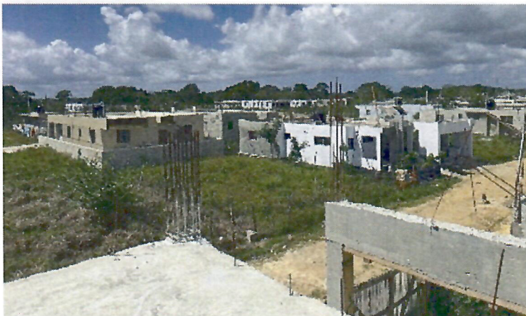
A view of the neighborhood being built next door as seen from the rooftop of the new church building.
